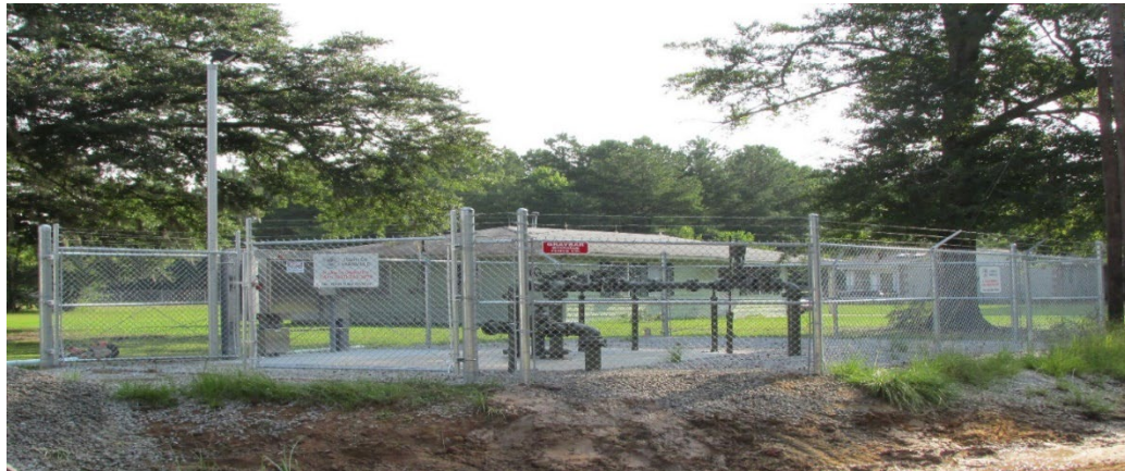
Mill Pond Lift Station
