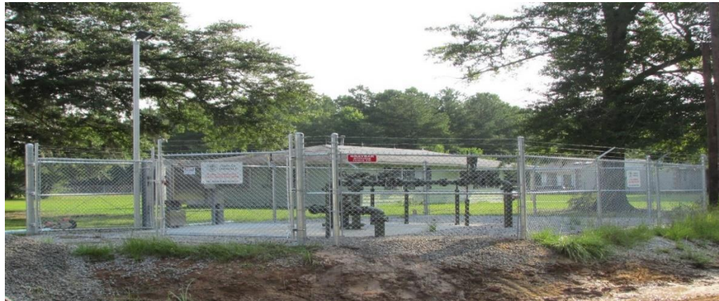
Mill Pond Lift Station
