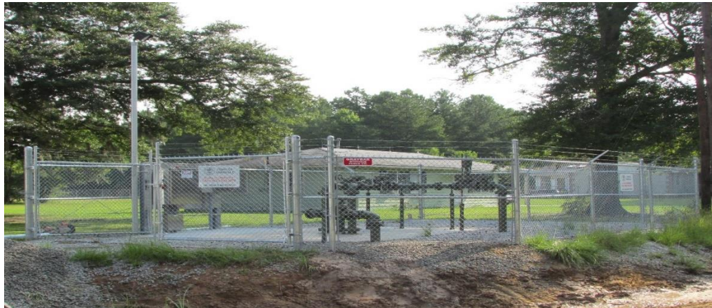
Mill Pond Lift Station
